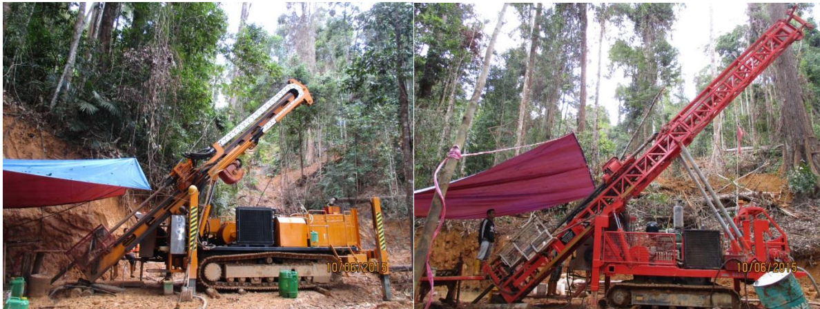
Figure 3.14 Chungwon D900 (left) and Sandvik DE710 (right) drill rigs
